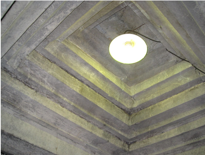
Figure 1-1d, Stepped caisson roof of the main chamber in the Baiji Tomb. Photograph by the author.
