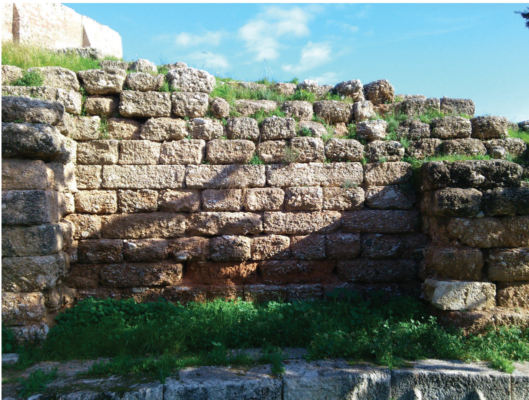
Figure 7: Retaining wall west of the auditorium of the Theatre of Dionysos at Athens (photo: P. Pedersen).
