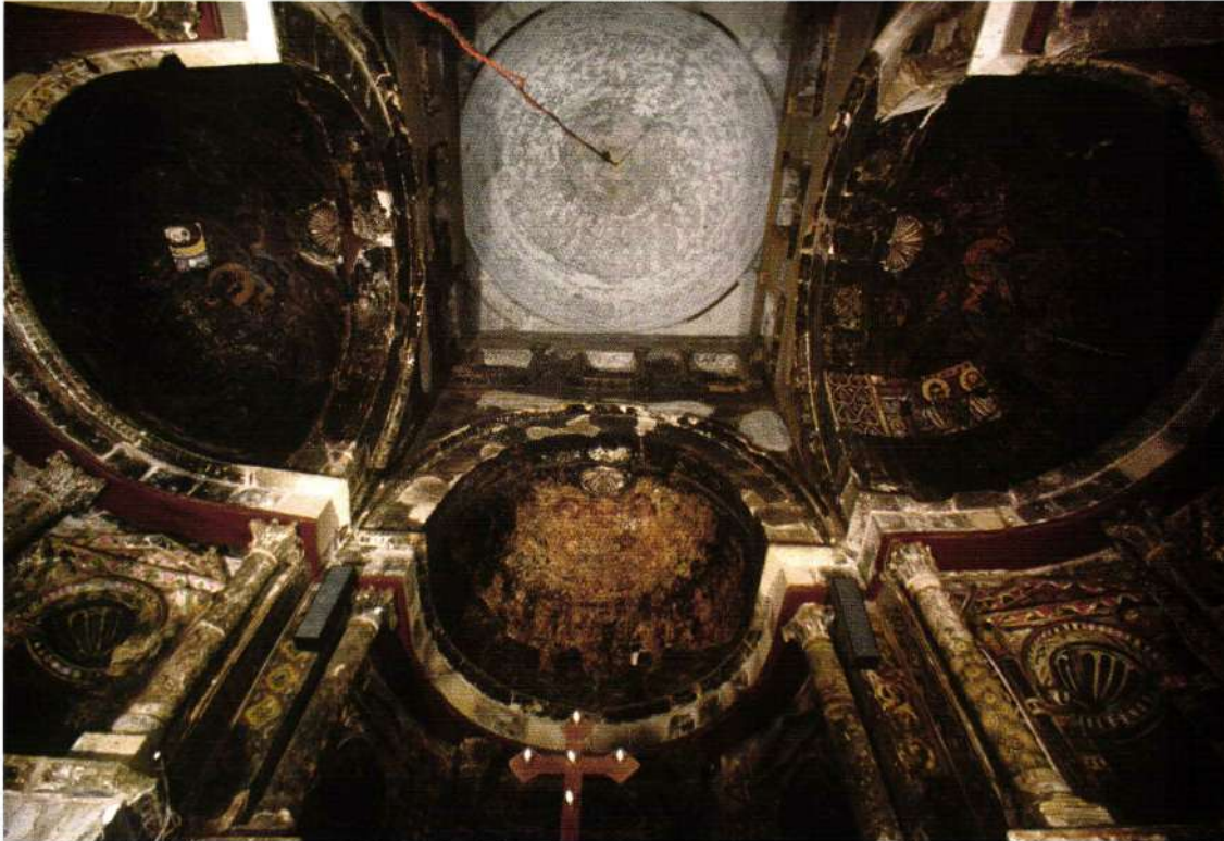
4. View looking up into the three apses of the Red Monastery Church Sanctuary, showing test cleanings in the north (Virgin Mary's face) and south (saints) semidomes. Photo: Patrick Godeau. EAP/RM March 2003
