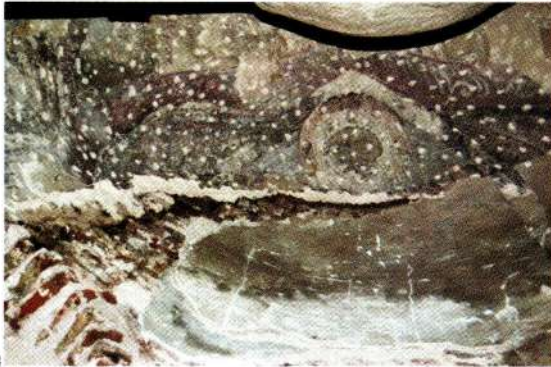
Figure 3. The central portion of the semi-dome before cleaning, showing Christ's head and the surrounding band of flames. A crack runs up from the left niche and across below Christ's head. Photo: Tim Loveless
