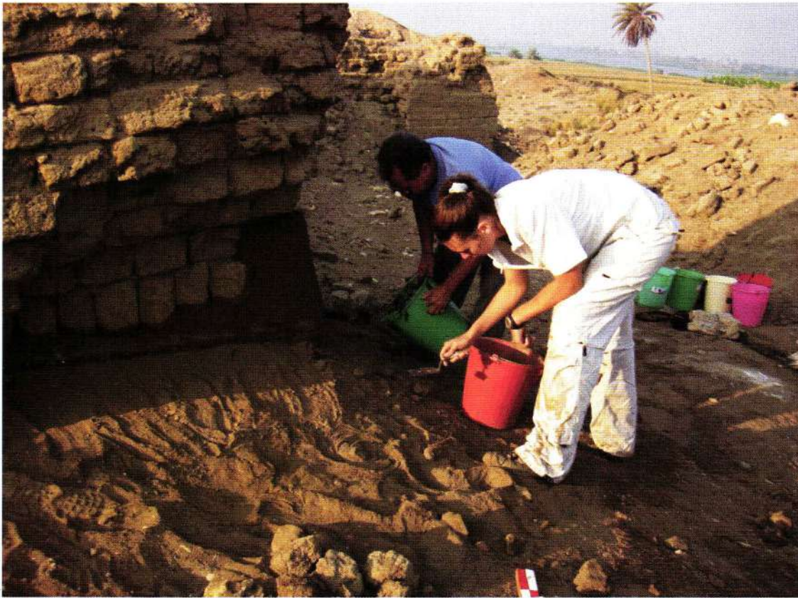
7. Maury Morgenstein and Malia Johnson putting the finishing touches on the cement and rebar support beneath a severely undercut wall on top of Tell El-Hibe
