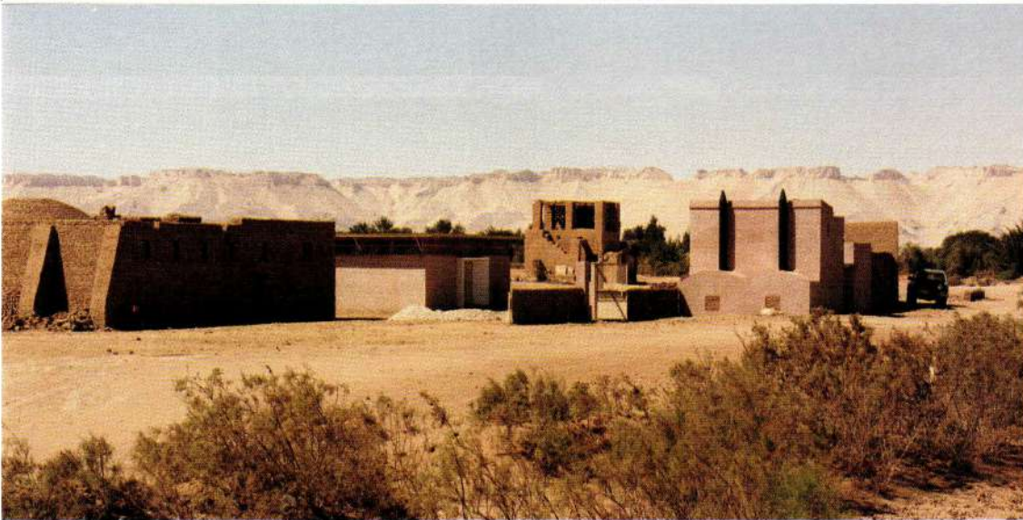
Site compound showing new composting toilets, conservation room and main work room to right, with replica villa of Serenus (under construction) and new block storage facility to left, and guard house at center. Photo: author 2009
