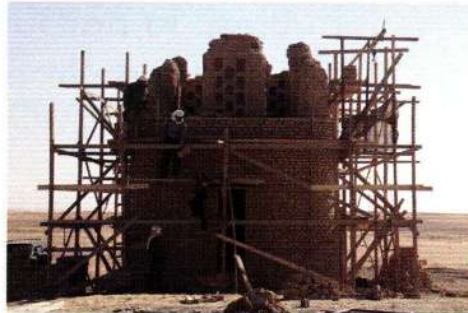
Fig. 7: The north wall in the process of rebuilding with the team energetically passing up bricks. Photo by S. Ikram, ©NKOS
