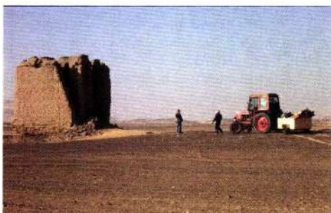
Fig. 5: The first triumphal arrival of the tractor and trailer with part of the scaffolding and the tools required for its erection and the restoration of the pigeon tower. Photo by S. Ikram, ©NKOS
