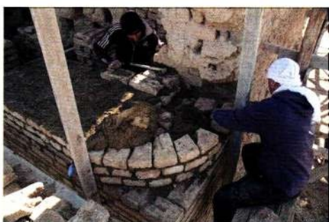
Fig. 6: The brick work being laid at the point where the tower's corners become rounded. Photo by S. Ikram, ©NKOS
