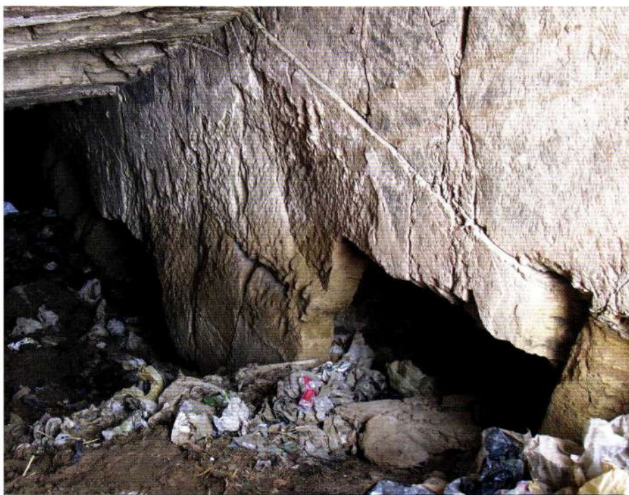
Figs. 2a and b: Hagr Edfu, 2010 and 2012 photographs of the north wall of the slopping corridor of the pylon "tomb," the stone of which is now disintegrating due to local irrigation systems that have caused the water table to rise. Photos by Lamia El-Hadidy and James Rossiter. For plan and report, see ARCE Bulletin 197–Fall 2010: 4–7.
