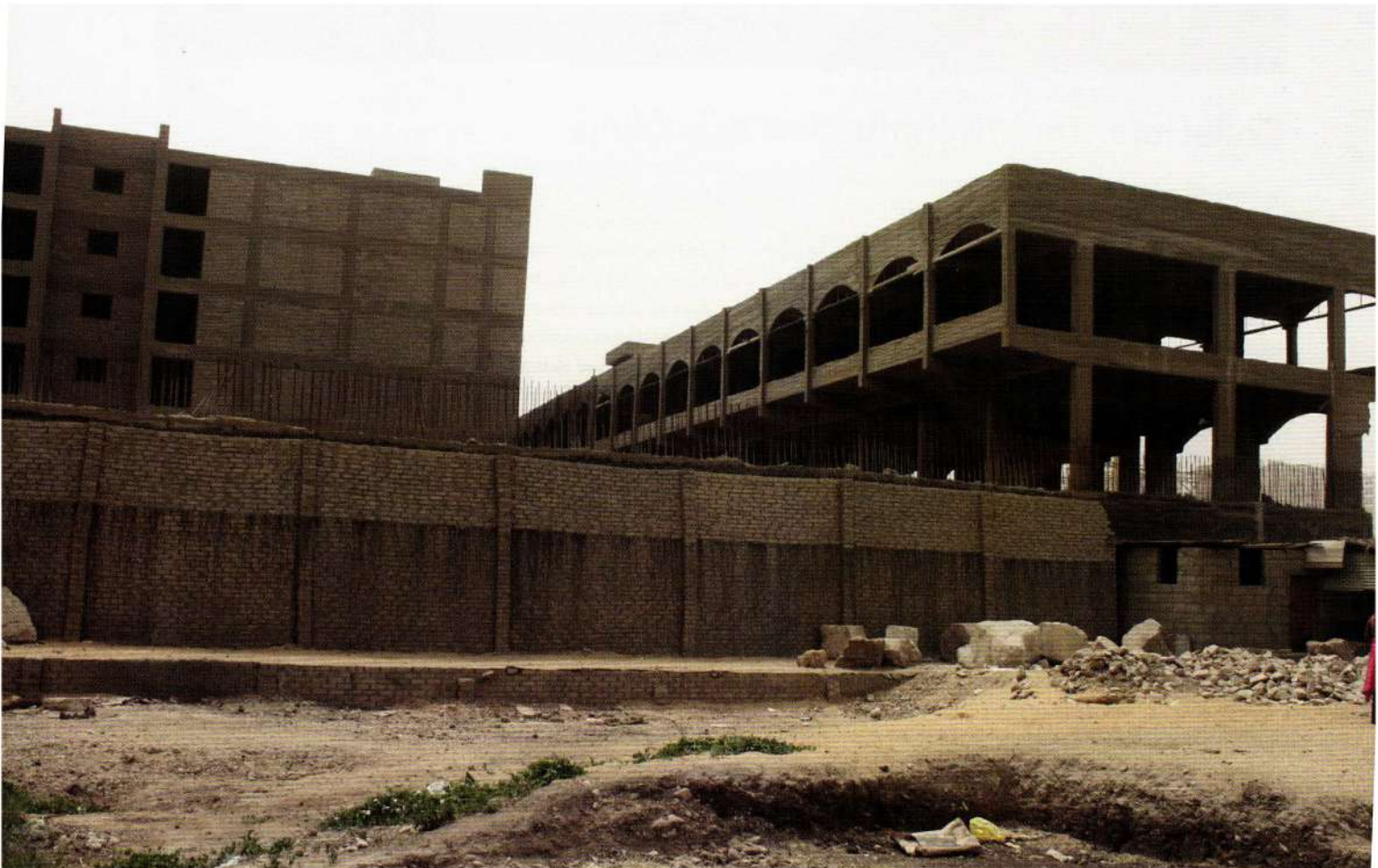
Fig. 1: Land grabbing at Al-Matariya, ancient Iwnw (Heliopolis), with large apartment buildings and shopping malls encroaching upon the archaeological site. Photo courtesy M. Hanna.
