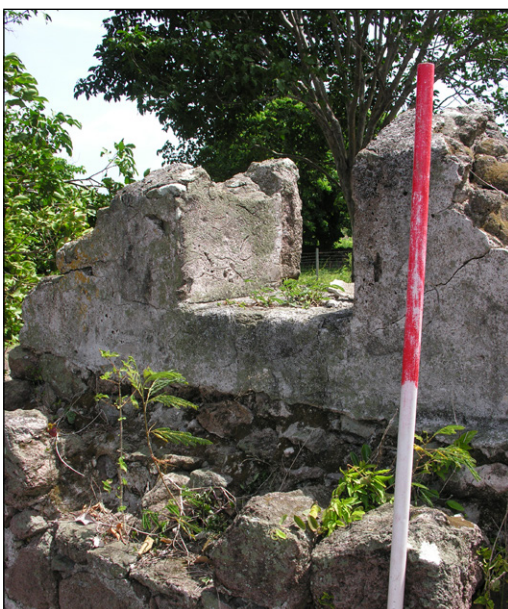
Figure 2.18. Fenton Hill: Structure A, E wall from outside showing window in gable and offset wall for gutter
