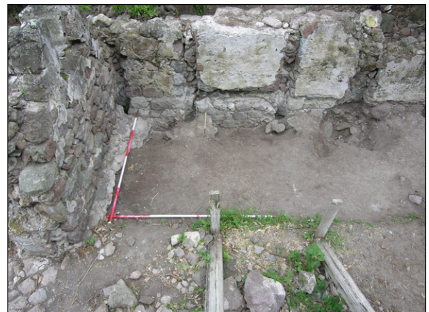
Figure 2.20. Fenton Hill: Structure A, S wall showing vertical slots 126, 114, 116, 112 (L to R), horizontal slot (125) and mortar line, from N
